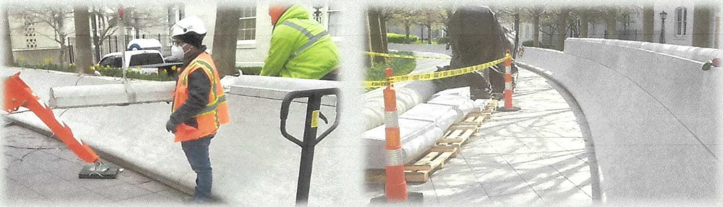
The original wall top-cap was removed and replaced with a more spacious and useful addition for names to continue to honor our fallen
